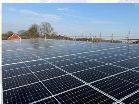
Roof-mounted solar panels in Aldershot (Aspire)
