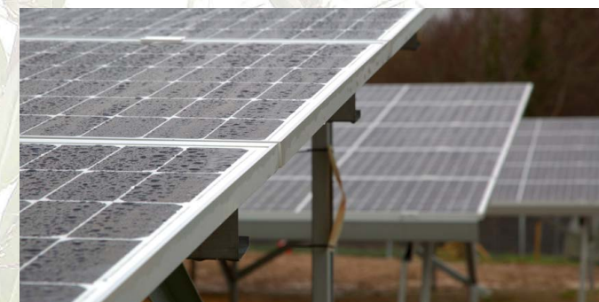
Ground-mounted solar panels at Larkhill Garrison (Aspire)
